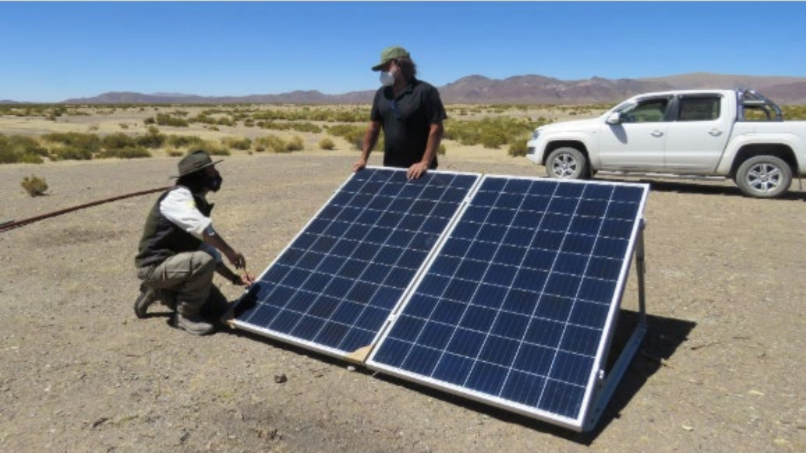
Solar water pumps installation in five ranches of the locality of Pasajes, Pozuelos Lagoon, Argentina
